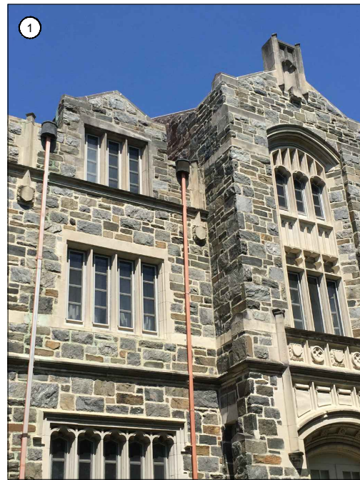
STONE/CAST STONE VENEER OF SIMILAR COLOR, SCALE AND PATTERN AS ORIGINAL 1913 BUILDING
